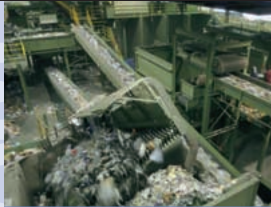
▲ Single Stream Installation Tide Water, USA. Capacity 20-22 tons per hour.
