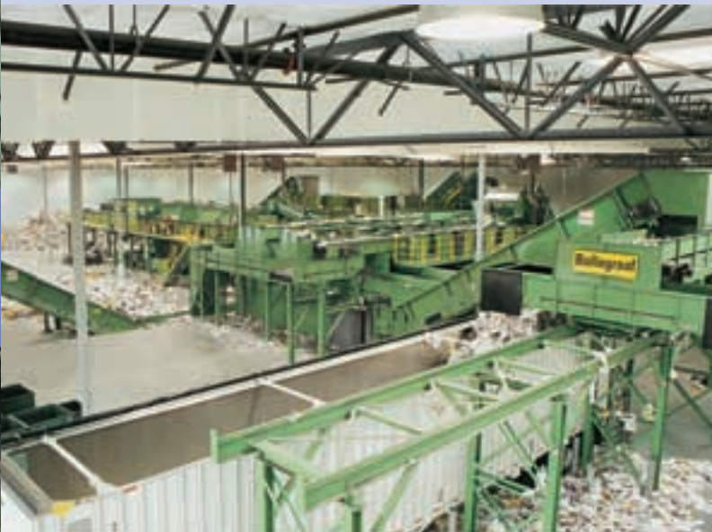
▲ Single Stream Installation SP Newsprint, USA. Capacity 15-20 tons per hour.
